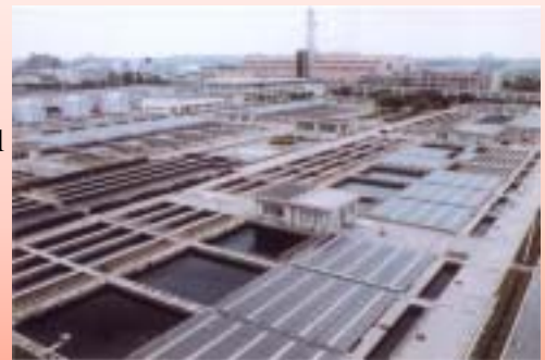
Facilities for generating photovoltaic power at the Murano filtration plant
